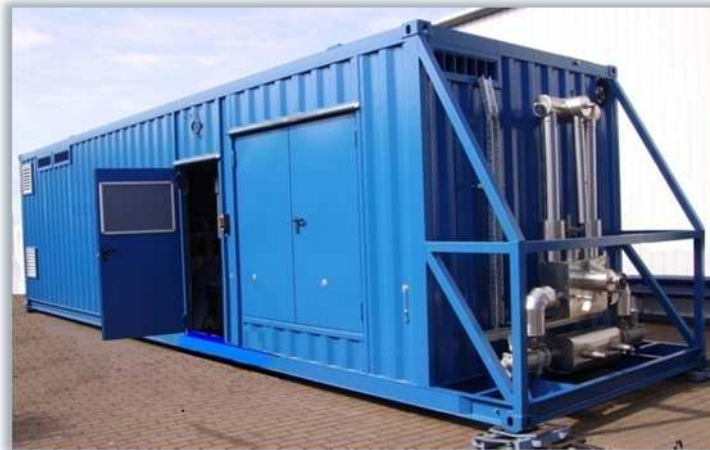
CO 2 / propene cascade refrigeration system in a container
