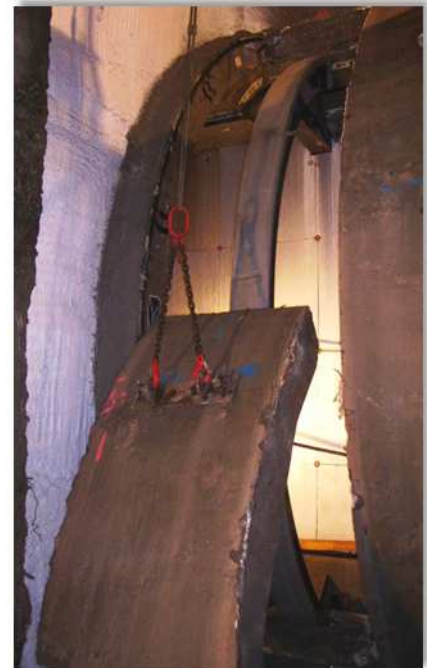
Frozen soil (white) surrounding a tunnel which has been opened under protection of the ice shield in order to be connected with an underground railway station.
