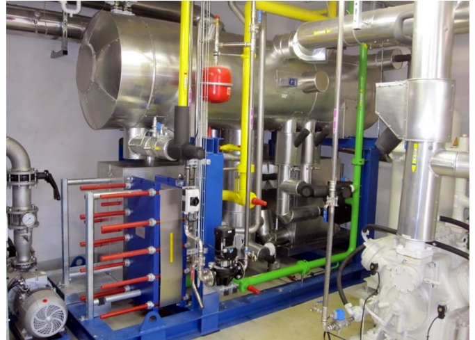
Fully installed separator unit in the machine room
