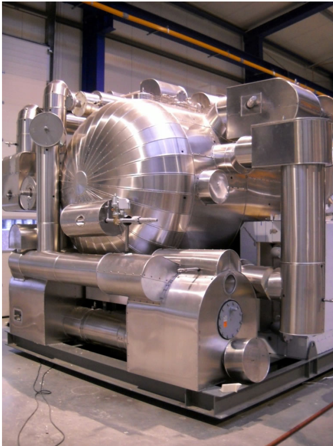
Assembly for cooling toluene to -72.5^{\circ}\text{C} during and after the completion of insulation work
